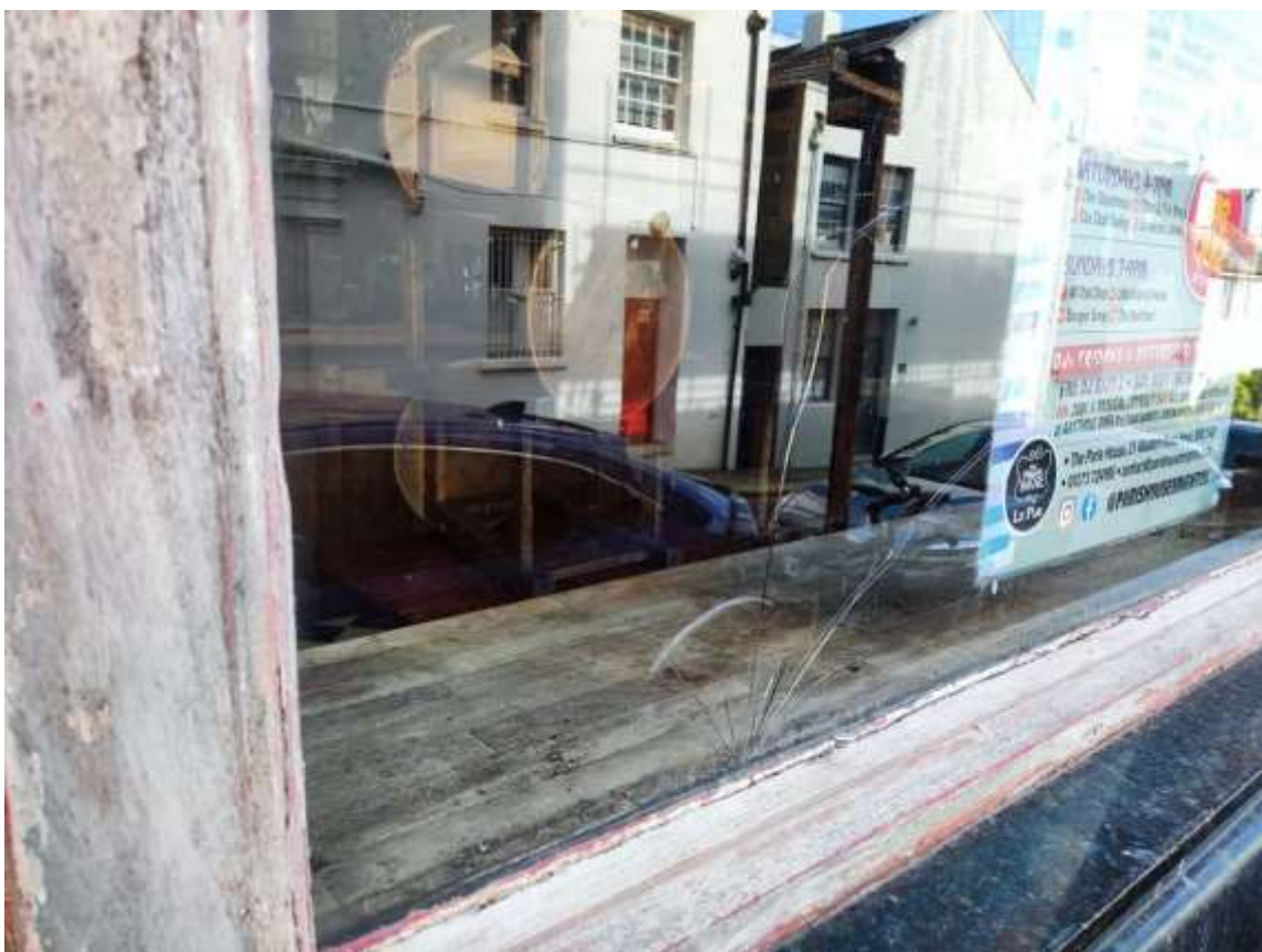
Figure 10: Glazing on Brunswick Street East façade is cracked
