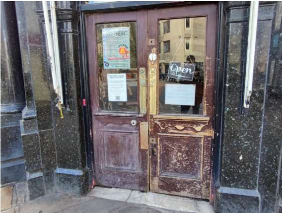
Figure 8: The entrance doors are in a poor state of repair and there is no lobby to reduce noise breakout
