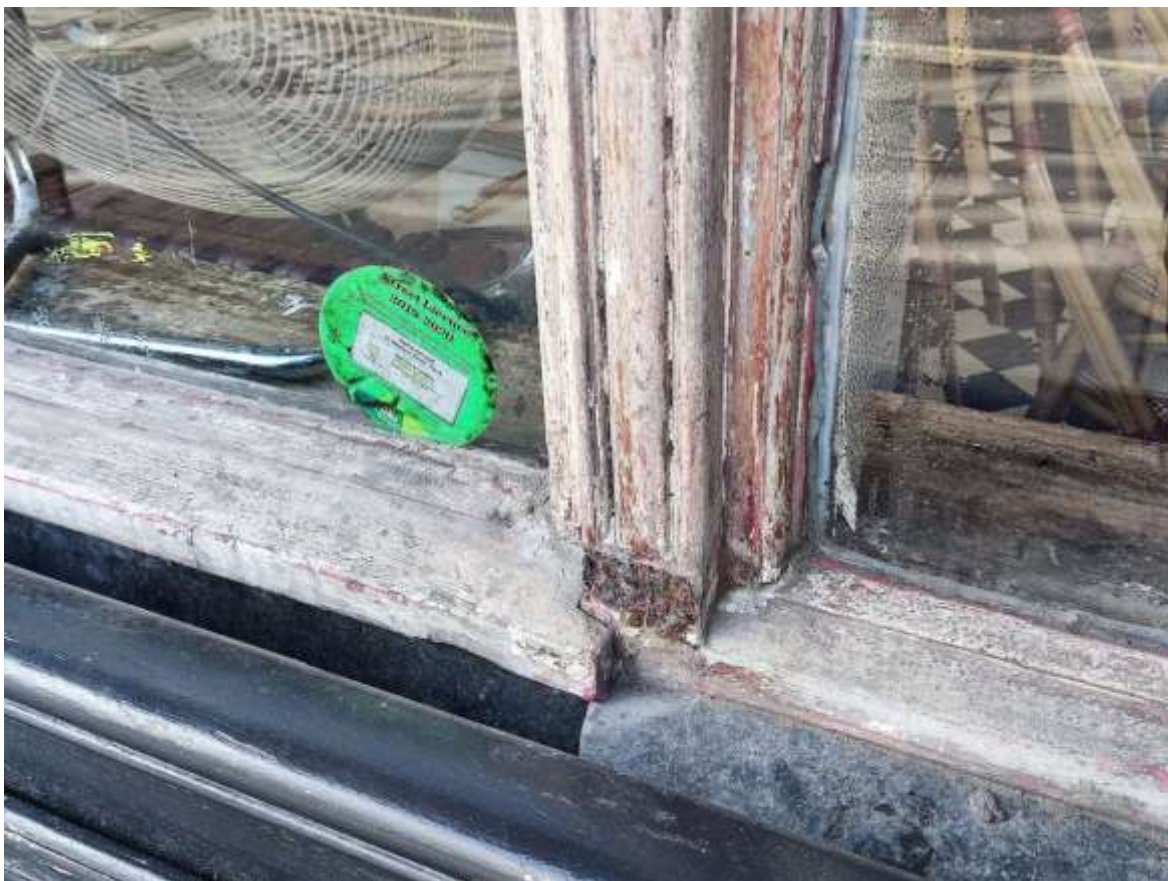
Figure 9: Glazing on Western Road façade. Frames are damaged and gaps are roughly patched silicon
